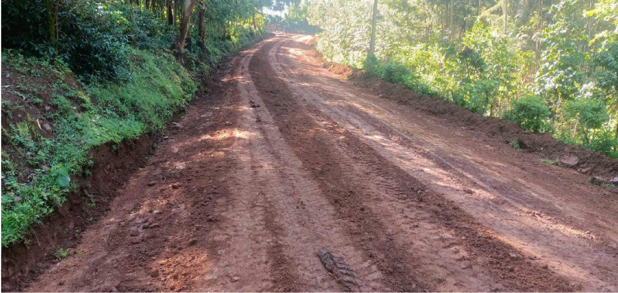
COMPLETED GRADED SECTION - SOUTHPORT VENTURES LIMITED [STAGE MILKA – MISAMBI SEC. SCHOOL ROAD]
